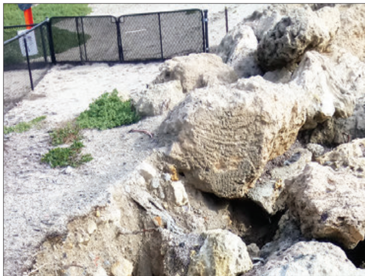
• Erosion of the sea wall at Rous Head. Photo supplied
